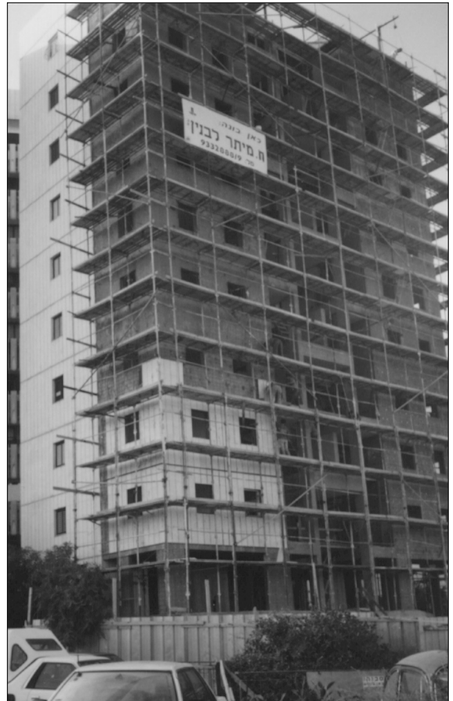
FIGURE 3. Enlargements in process in Tel Aviv. The households continued living in their apartments while the construction work took place.
